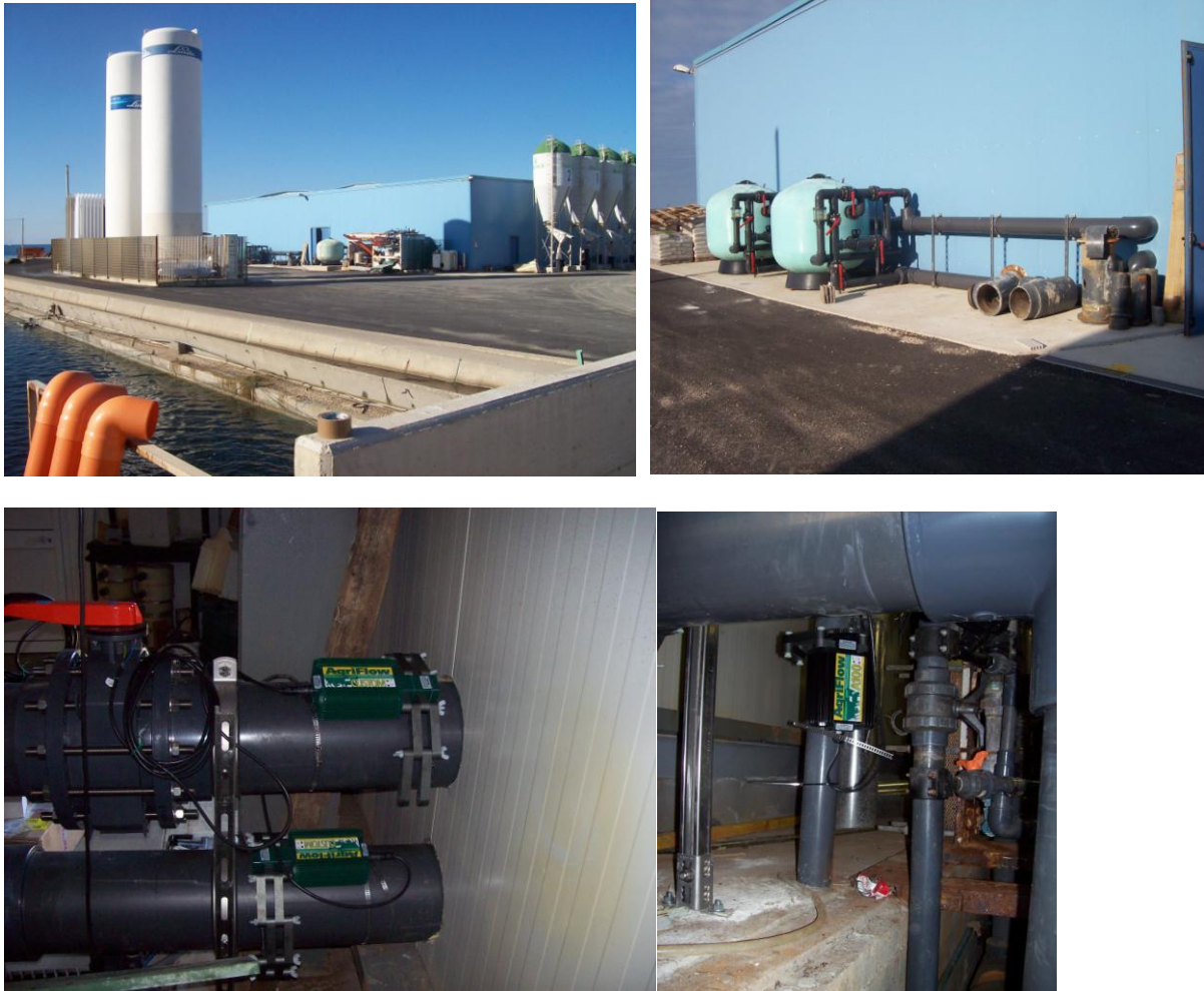
Figure 3: Installed Agriflow units
