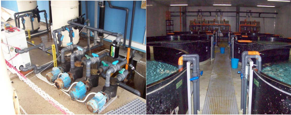
Figure 4: The Pump set feeding the hatchery, with an Agriflow A60 installed (left), and the breeding tanks (right)
