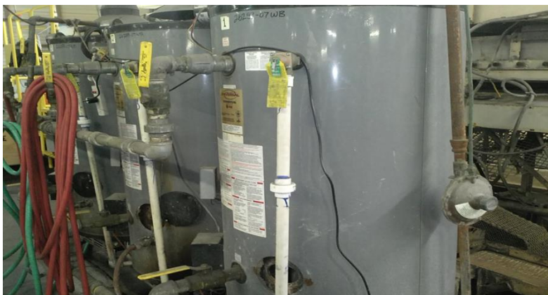
Three water heaters in parallel
